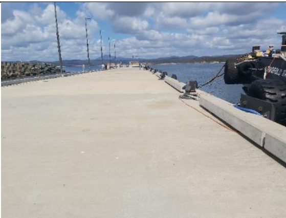
View of the wharf extension with the moored tugboat. Noted that the tugboat is connected to shore power.
