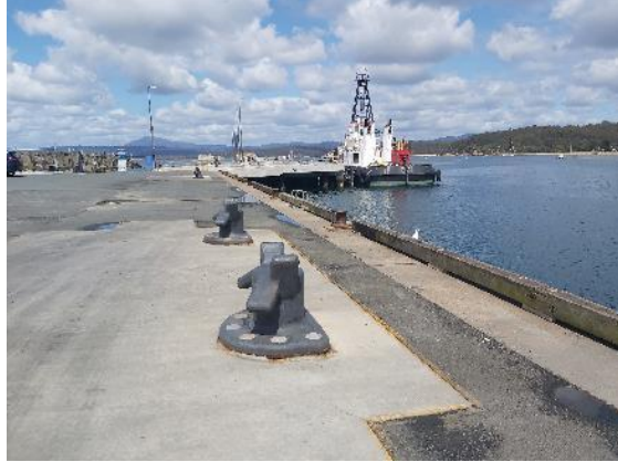
View of existing breakwater wharf, showing new mooring bollards in foreground and wharf extension further on.
