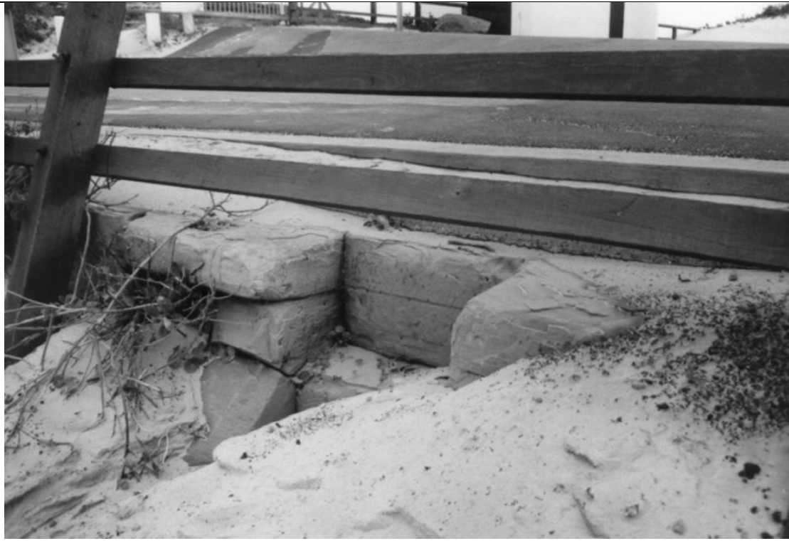
Caption: Top of sandstone steps, with newer timber balustrade running over top.
