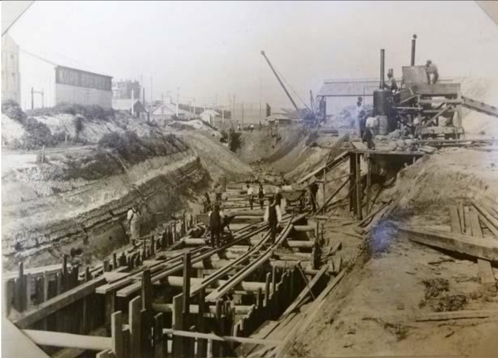
Caption: View of what appears to be the conversion of the west section of the cooling water canal to a conduit
